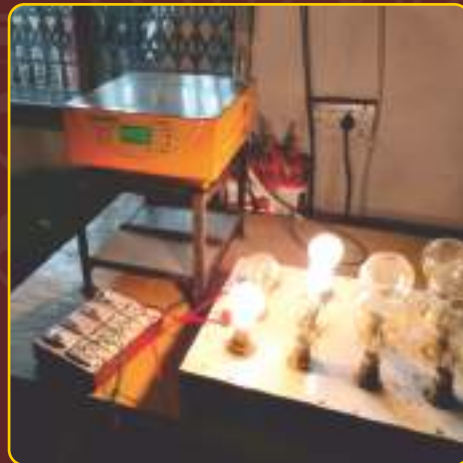
Battery ,Solar inverter and load
